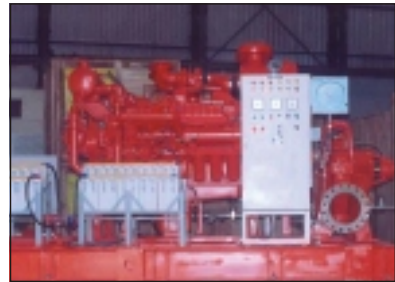
3 X VTA - 1710 F3 Dolareh Bulk Terminal Project, Sharjah
